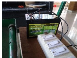
Figure 4: Battery and Control switches
